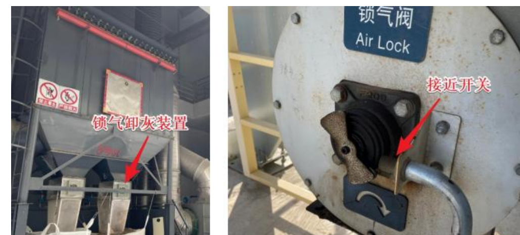
锁气卸灰故障监测
